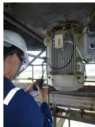
Motor on cooling Fin-Fan
